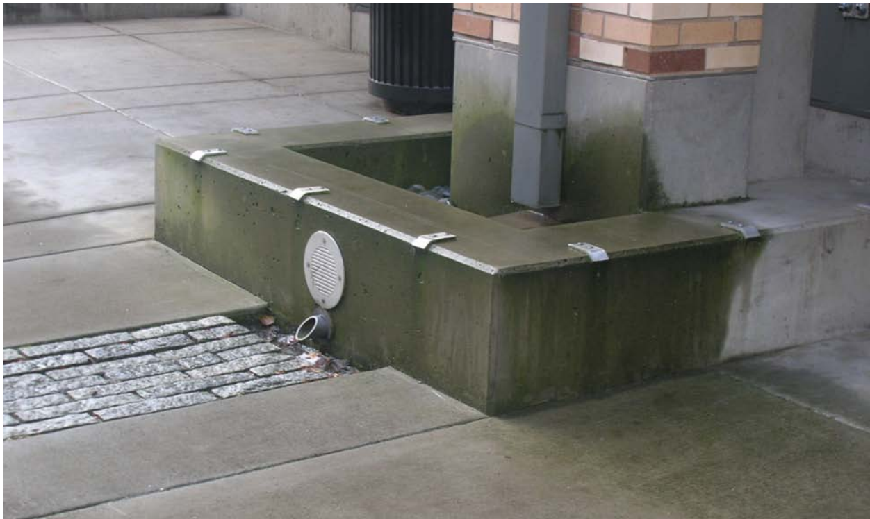
Fig. 6. Detail of the downspout system and its connection to the runnel across the alley
