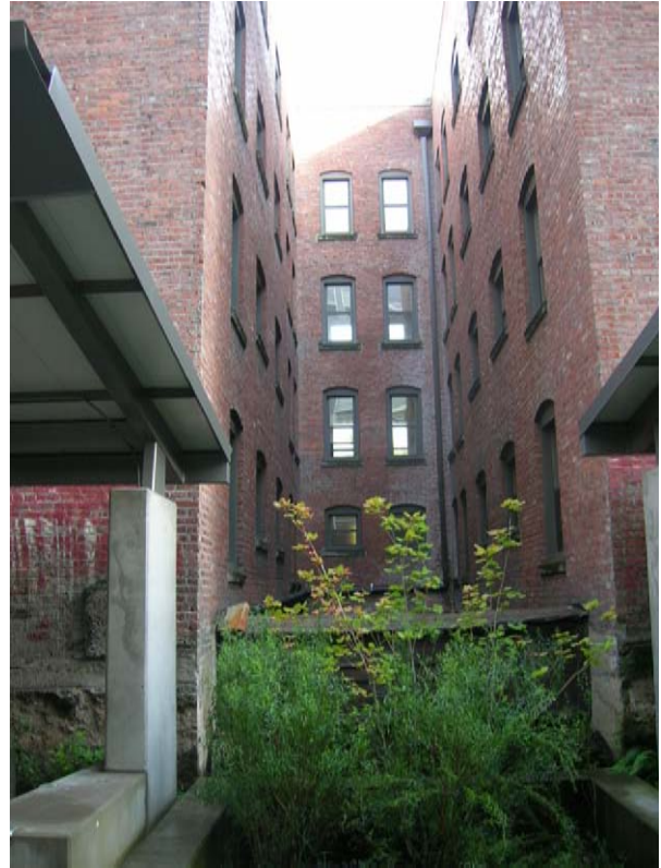
Fig. 5. The connection between Epler Hall and adjacent King Albert Hall across the "bio-alley"
