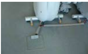
Data connection for cardio machines at WOU.
