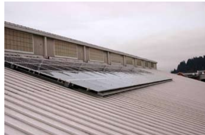
Photovoltaic panel on the SRC roof.
