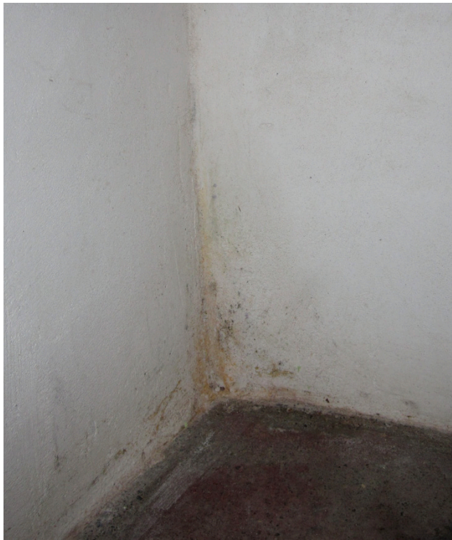
Fig. 1: Mold growth on shower wall
