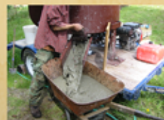
This mix was later poured (crudely) into the stick-framed walls and floor of an older structure for insulative purposes.
