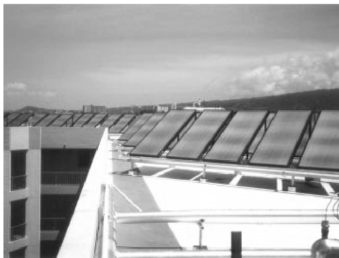
solar hot water panels on Banyan Street Manor, a fifty-four unit apartment building in Honolulu, Oahu
