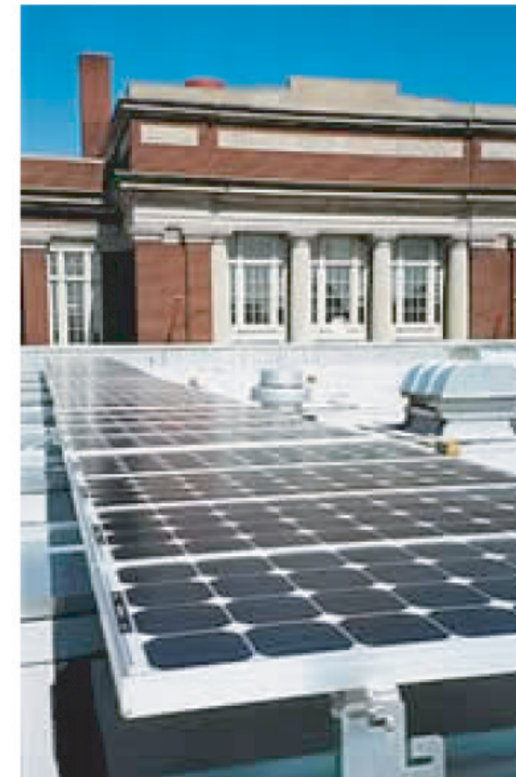
Internet image of roof-mounted PVs
