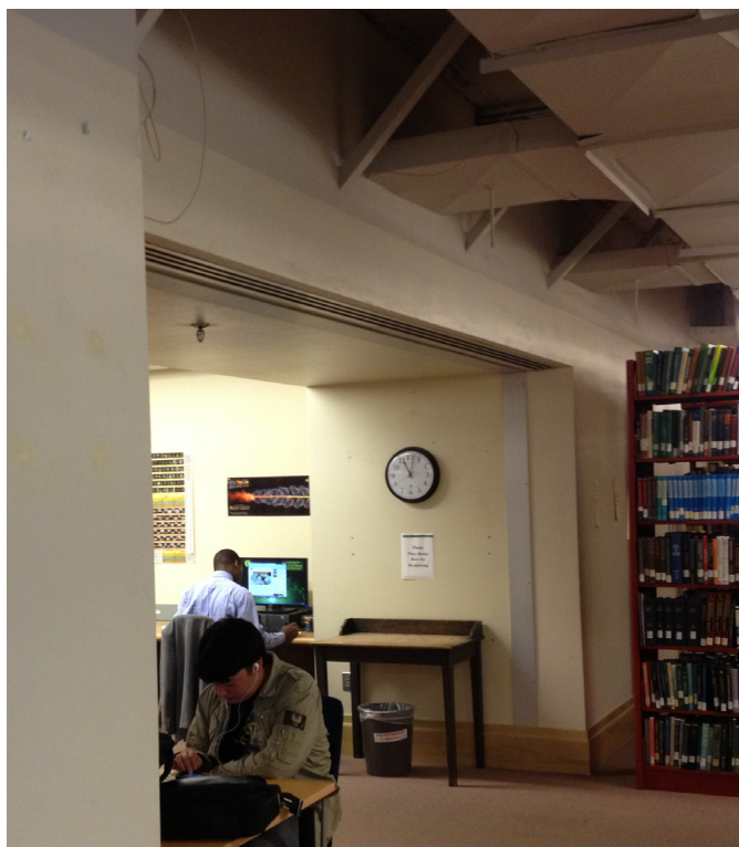
Deluge Curtain at Cascade Hall and Science Library Basement
