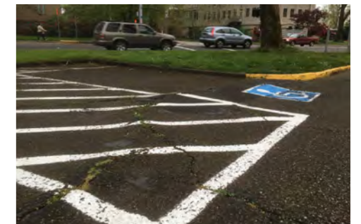
Before: Cracked pavement causes potentially unsafe conditions on campus
